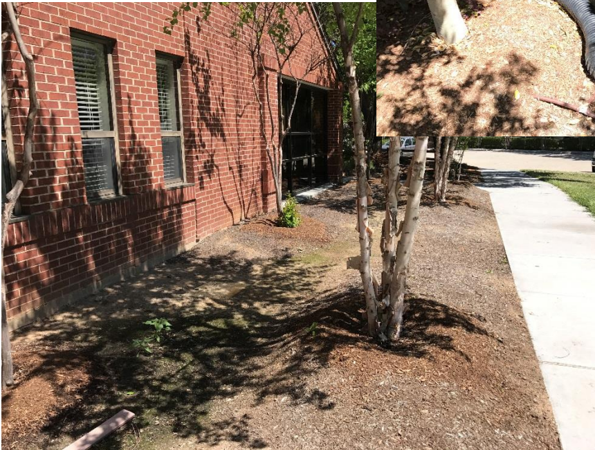
Images of drainage issues near structure
