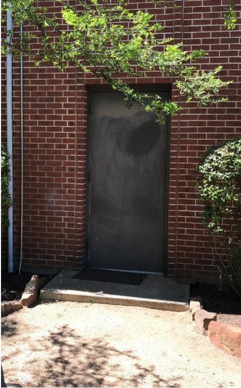
Non-ADA compliant exit
