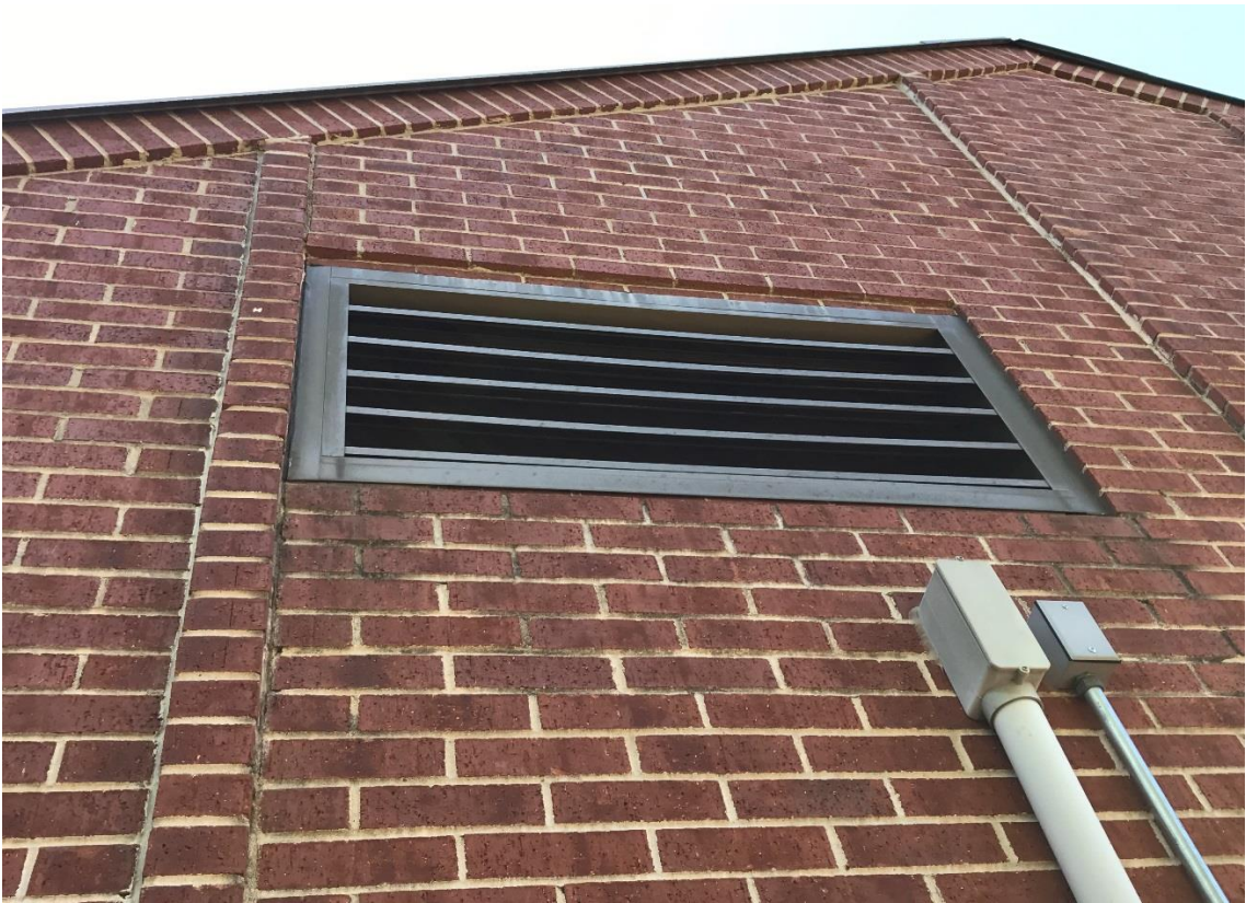
Mildew growth and sealant failures.
