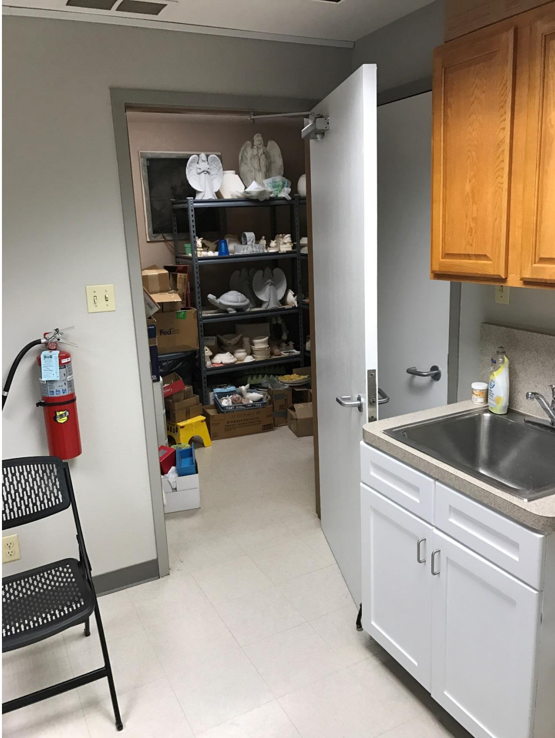
Ceramics – Non-ADA compliant doors & sink
