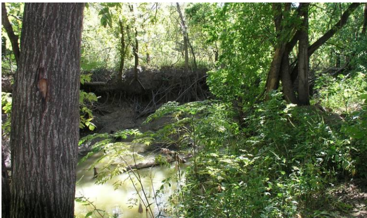
The creek bank exposes tree roots and the vertical edge appears unstable, caused by excessive flow and velocity. Plantings, once established, provide stabilization.
